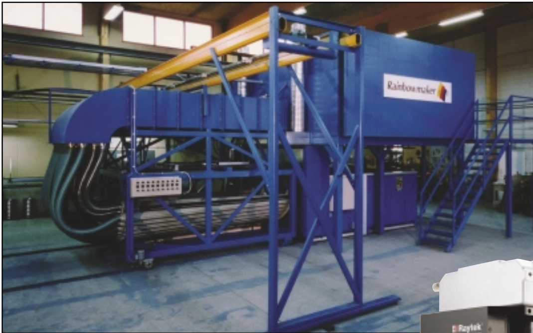
The GS100 provides real time temperature analysis for glass bending processes (Photo: Courtesy of Glassrobots OY, Tampere, Finland)
